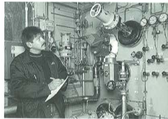
A Linde employee inspects the air separation unit at the Düsseldorf parent plant.
