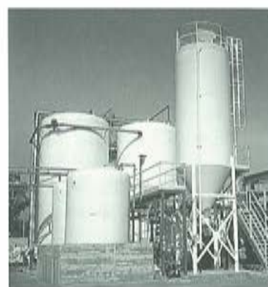
Tanks and lime silo of the new wastewater treatment plant in Barcelona.
