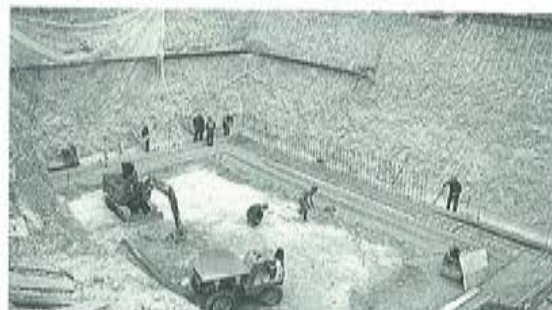
Reims: Additional collection basins increase retention capacity.
