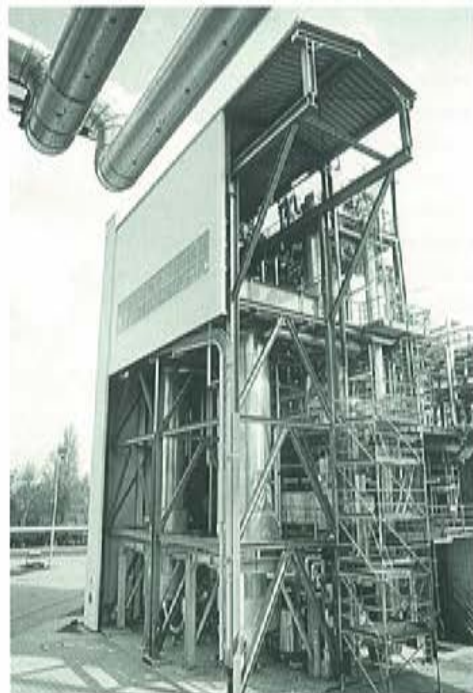
In operation since 1993: the world's largest hydrogenation facility for fatty alcohols in Düsseldorf.
