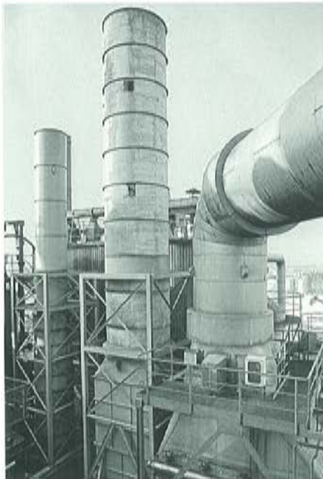
Five metric tons in weight and six meters high: the damper that was fitted to a detergent spray tower in Düsseldorf 1993.
