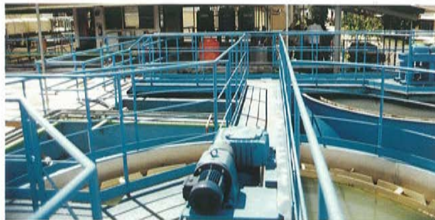
Henkel Indonesia's wastewater treatment systems are in perfect working order.
