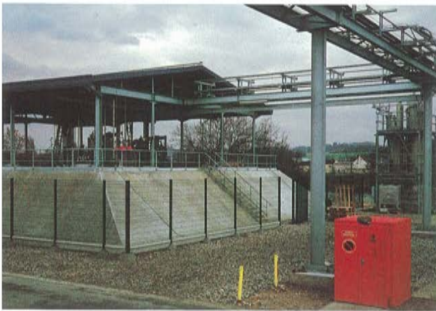
The new ethylene oxide tank farm at Sidobre-Sinnova in Meaux is equipped with sophisticated safety systems.
