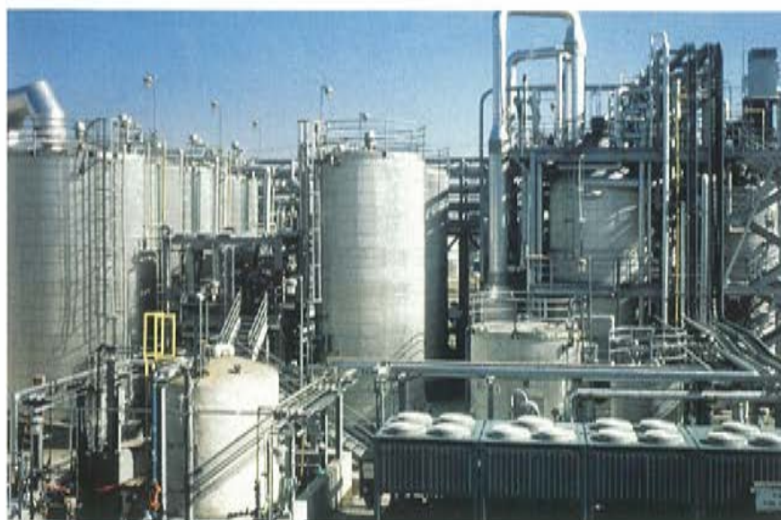
Production at near-zero emission rates: the alkyl polyglycoside plant in Cincinnati.
