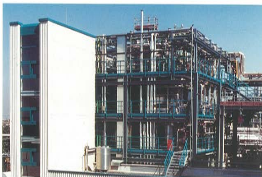
A world first in the Düsseldorf "oil quarter": the continuous fatty acid hydrogenation facility.
