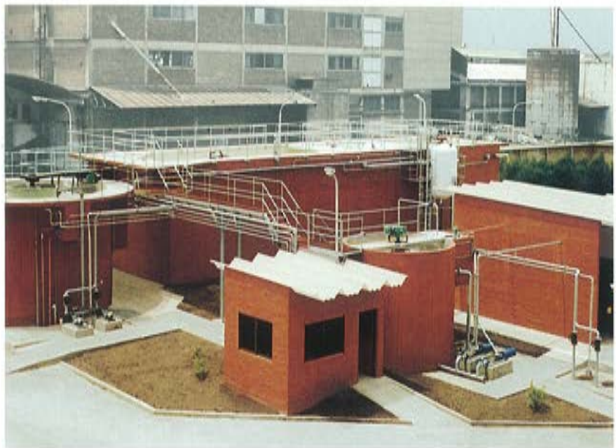
The new sewage treatment plant at Avellaneda can handle about 150 cubic meters of wastewater each day.
