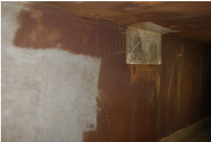
Photo taken in 2015 before coating with Loctite PC 7255 shows steel corrosion due to sulfuric acid.
