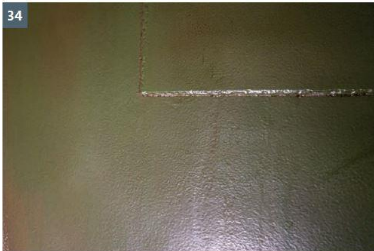
Inspection in 2020: minimum changes in color and coating thickness demonstrate the resistance of Loctite PC 7255 after five years of continuous use in extreme conditions.
