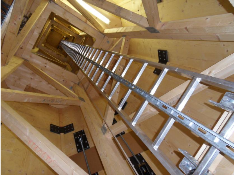
Internal view of the cross-laminated timber (CLT) panels used to build the TimberTower.
