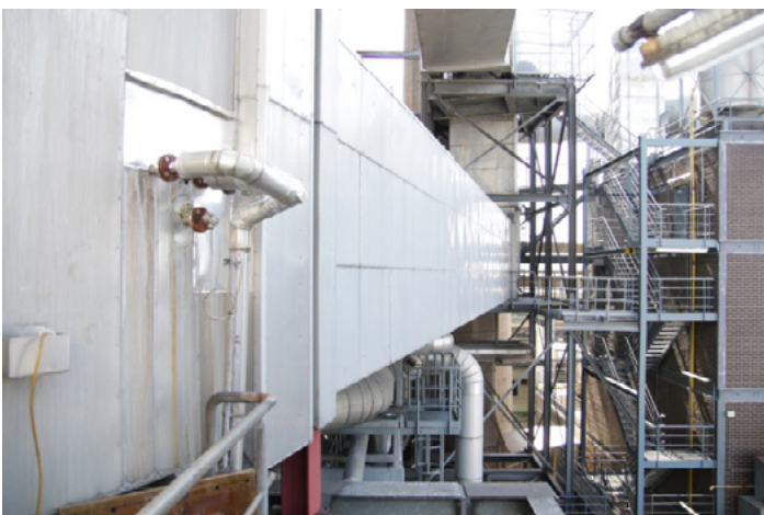
The flue gas duct viewed from the outside
