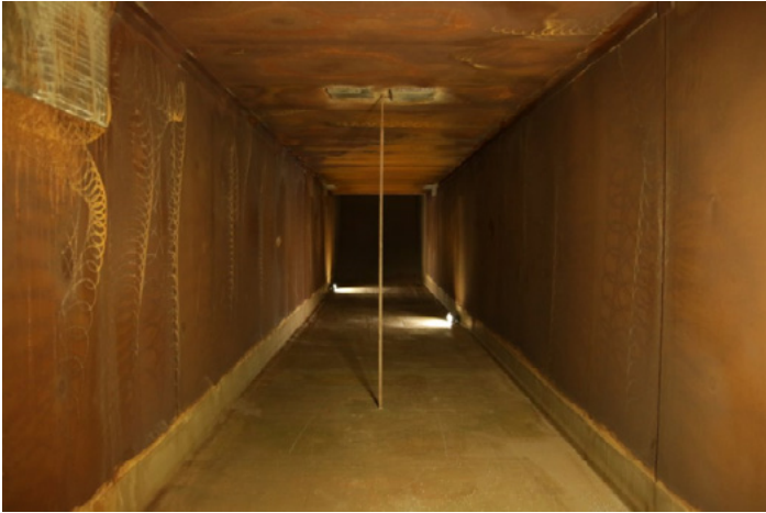
The flue gas duct of the site's own power plant after cleaning but before coating
